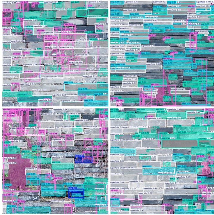
Figure 6: Defect detection and segmentation results
