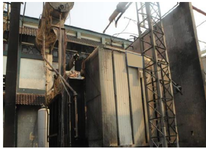
Fig. 3. Power transformer failure due to hydrolysis
