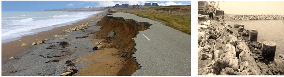
Figure 1. Examples of coastal erosion and abrasion due to waves
